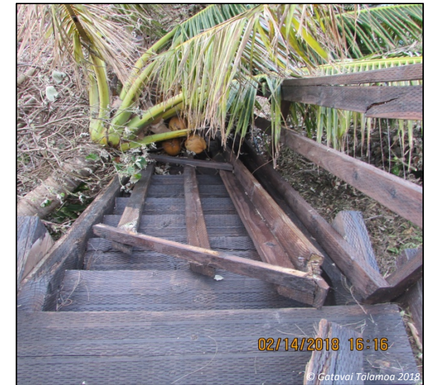
Cyclone Gita Damage at SMO February 2018
